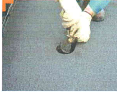
4. Leave the waterproofing membrane to cool for a few moments, then carefully cut out the hole in the rainwater outlet.
