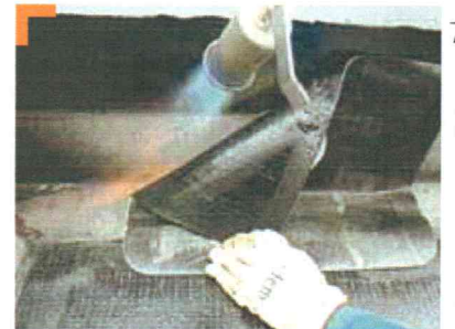
2. Weld the layer onto the first horizontal layer and against the angle already in place.
