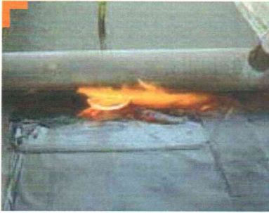
3. Lay and weld the second layer of waterproofing, covering the Depco opening completely.
